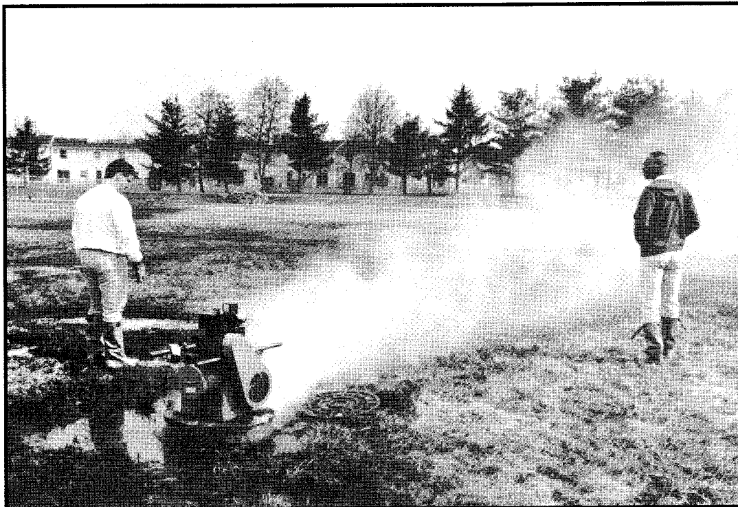
Contractors for the Public Works Department conducted delayed smoke testing of under-ground sewer line.
