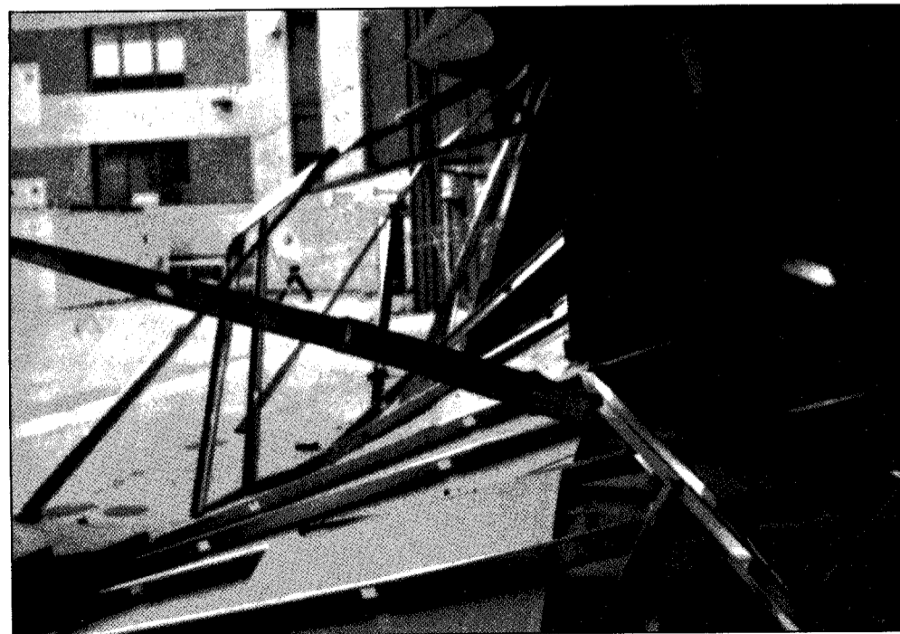
Accidents here are rare but a contractor's temporary hangar-door wall recently blew down. No one was hit but Mike Masington, Code 092, the Command Safety Officer, notes too often people pass this area reading while they walk; bumping into people and parked forklifts.
