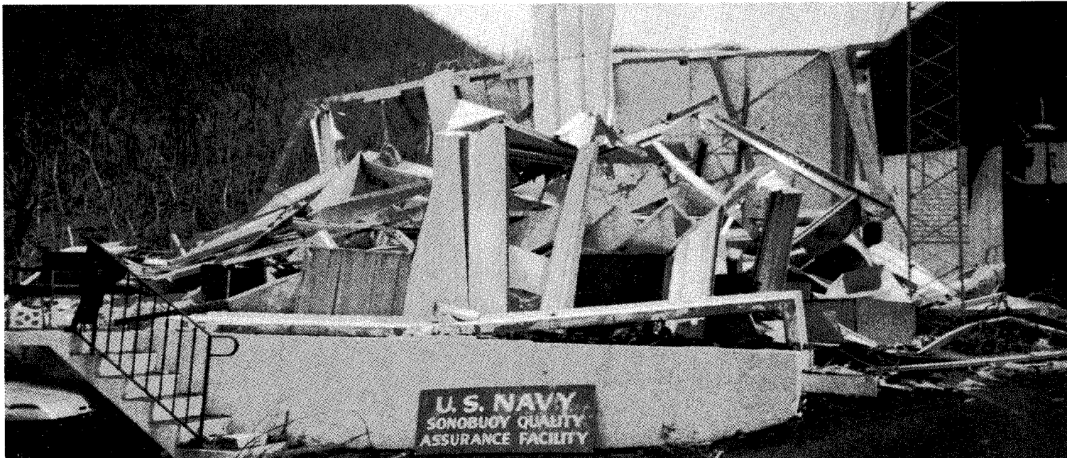
Front view of the Naval Avionics Center (NAC) Ham's Bluff test facility at St. Croix. The facility was used to test production sonobuoys (see add'l photos page 4).
